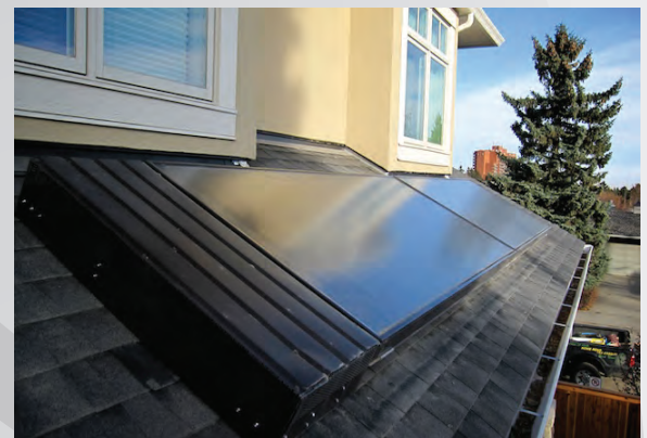
2 Collector Viessman system - Calgary, AB
