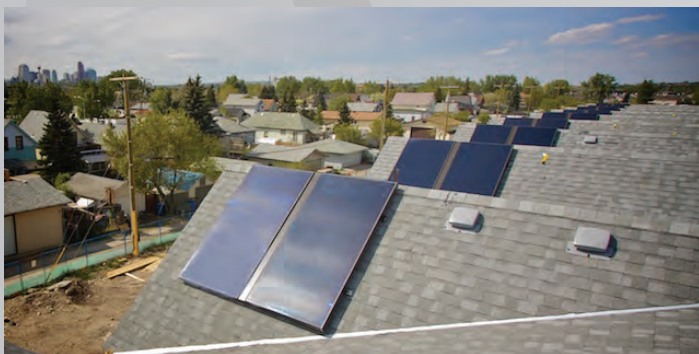
2 Collector EnerWorks systems - Calgary, AB
