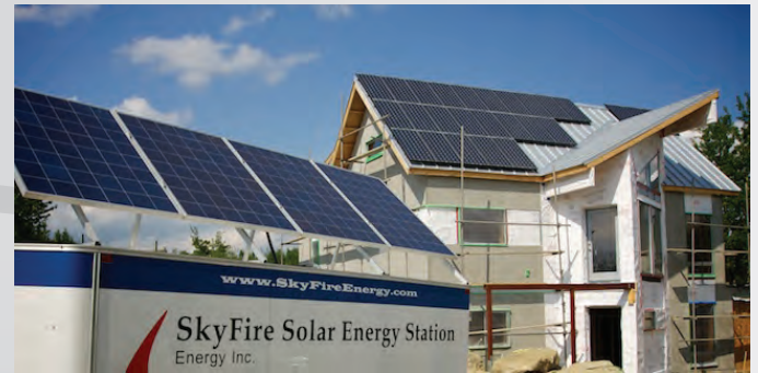
Echo Haven net-zero home 5.46 kW system - Calgary, AB Construction site powered by SkyFire off-grid solar trailer
